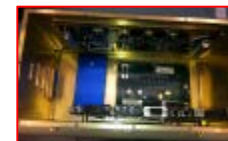
Power Control Unit (PCU)
